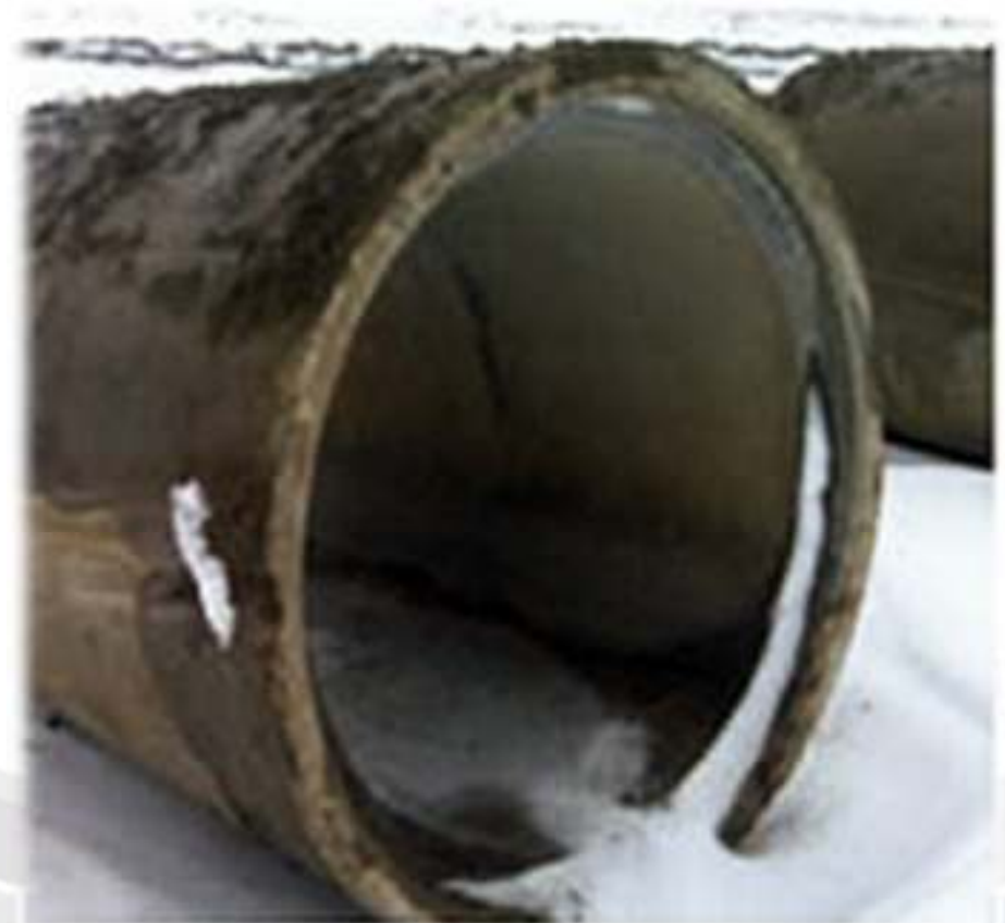
Thirty year-old 1350 mm diameter RCP ready for reuse as a storm sewer.
