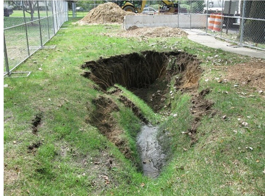
Sink hole along the HDD alignment
