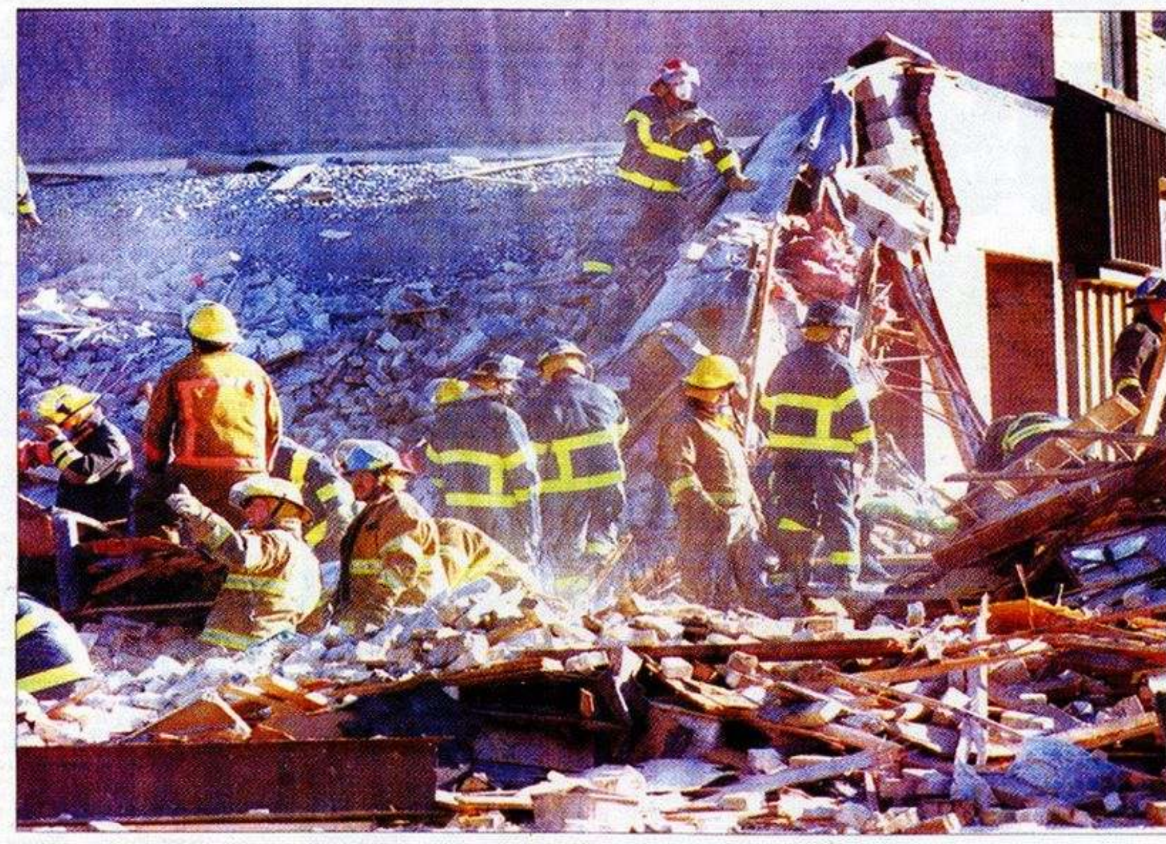
Firefighters from five surrounding departments combed through the rubble of the Bellantti's Pizza building Friday afternoon looking for victims from a fatal gas main explosion that leveled the building and heavily damaged adjacent structures.
