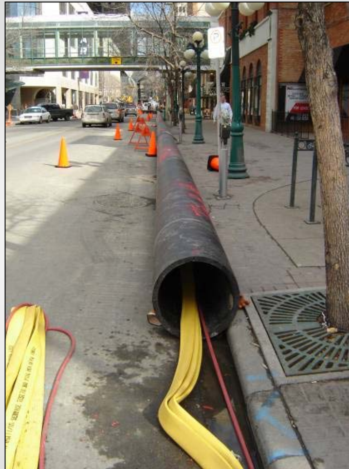
Supply air hoses and lubricating hoses installed inside replacement pipe from rear to bursting tool
