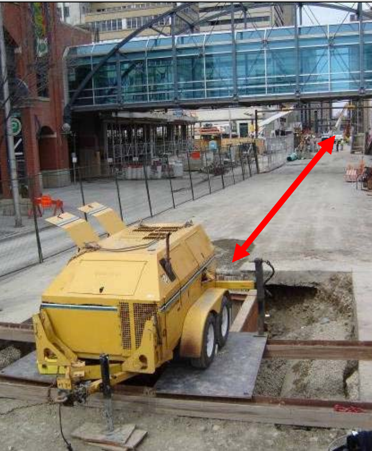
Constant tension cable guide winch over pulling pit. Red line indicates pipe bursting path
