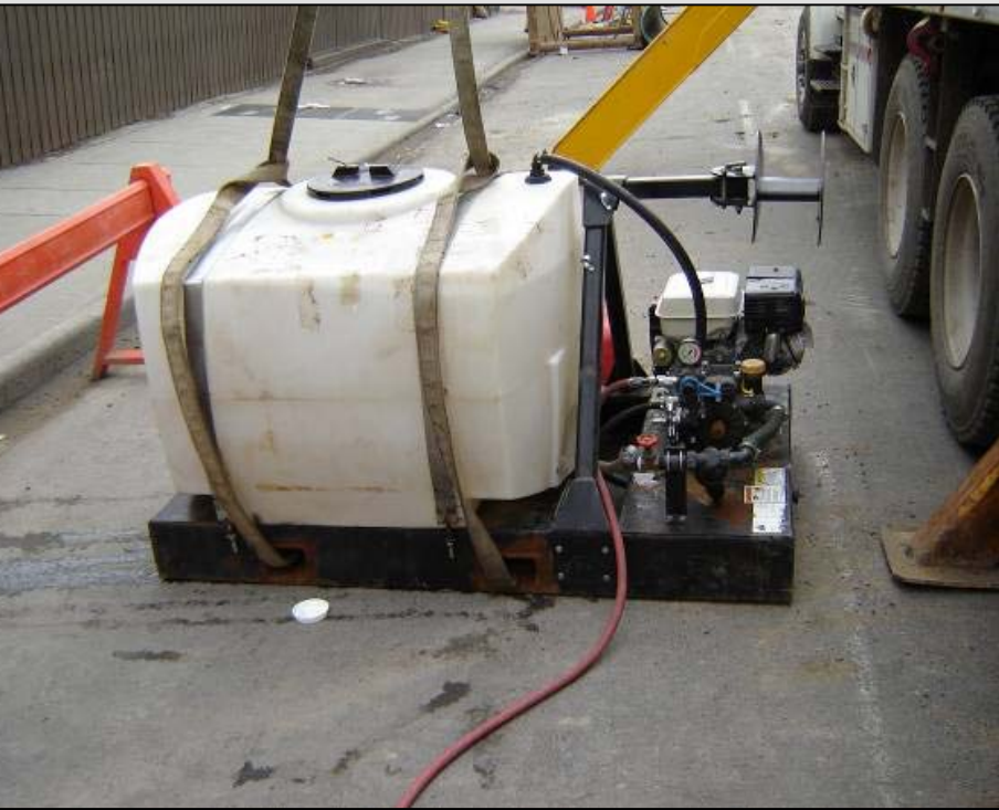
Lubricant mixing tank and delivery pump
