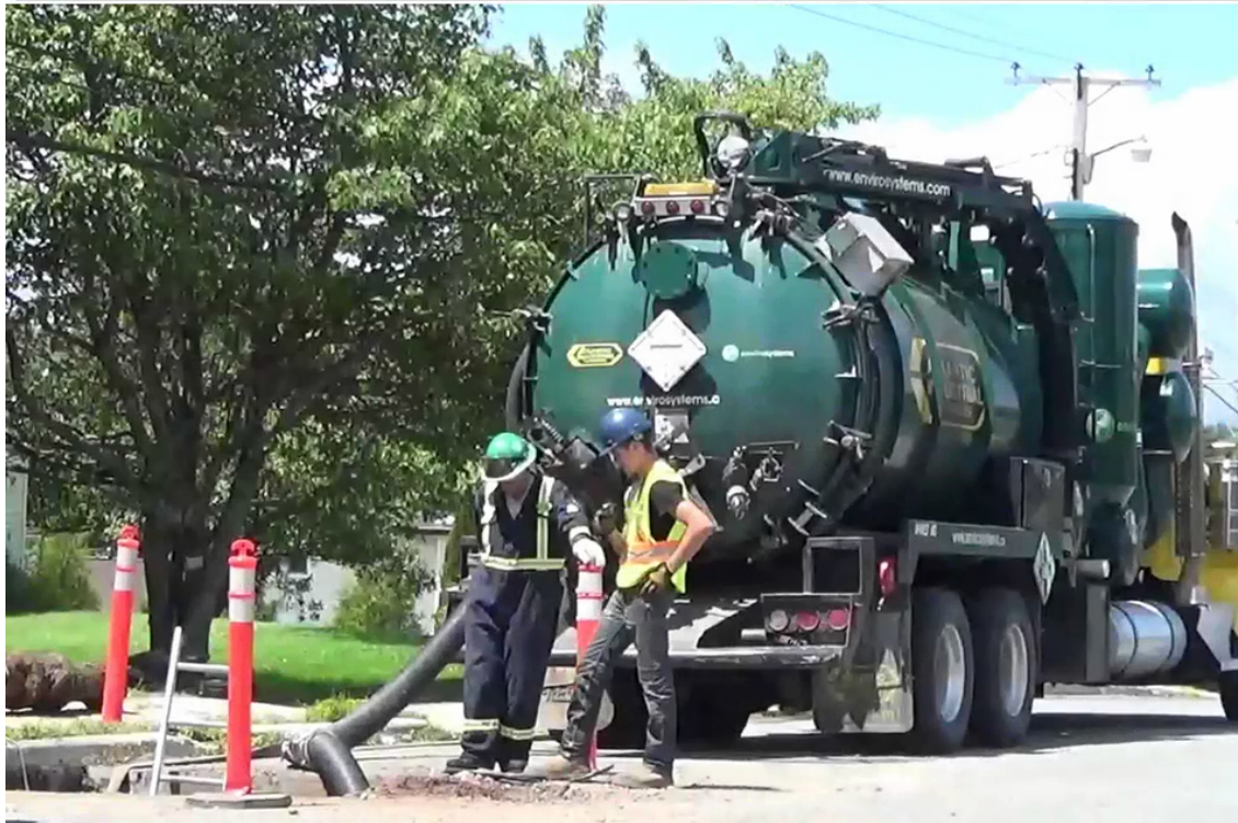
Trenchless Watermain Rehabilitation - Tomahawk™ Cleaning 150mm - 120 meter long watermain - cleaned and prepared for lining in 2 hours
