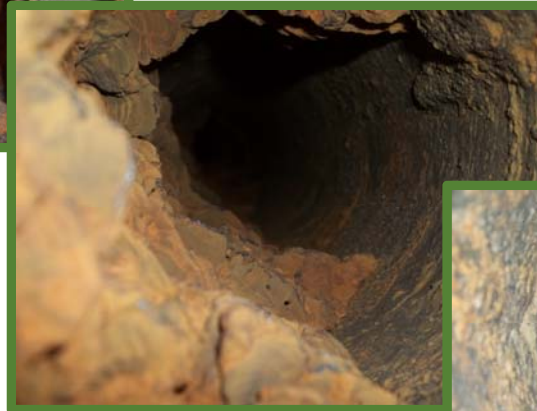
Partial tuberculation removal
