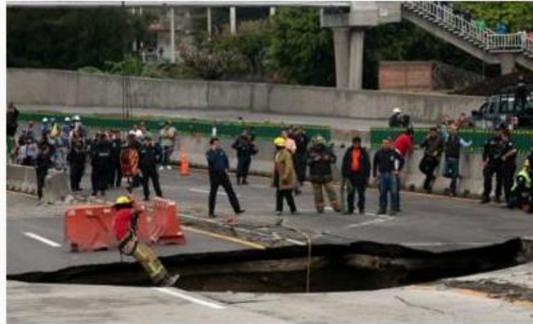
The sinkhole that appeared this morning.
