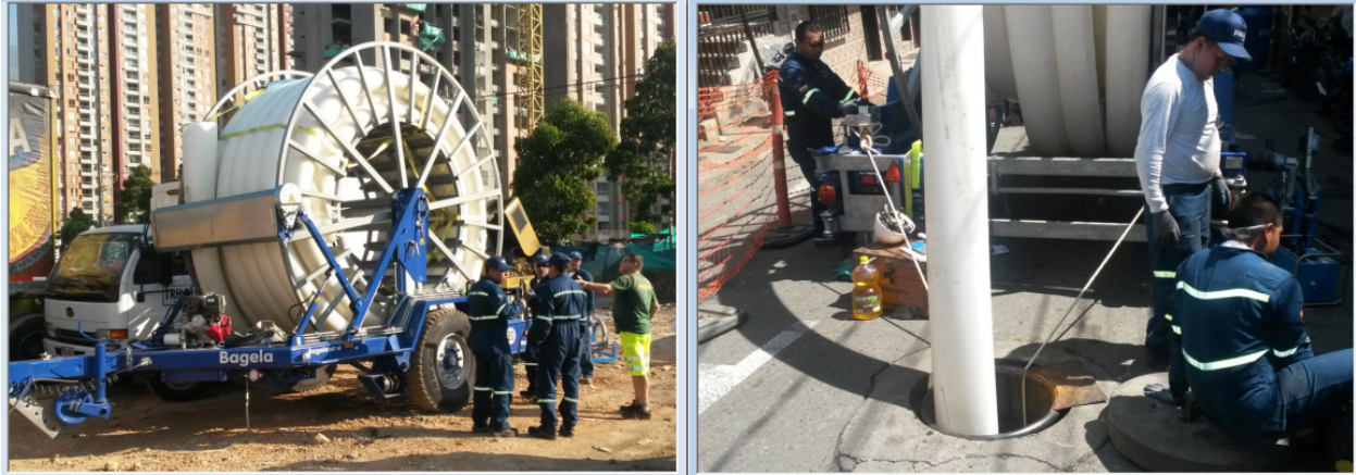
Figure 5 - Some impressions of the installation of Compact Pipe in the first project.
