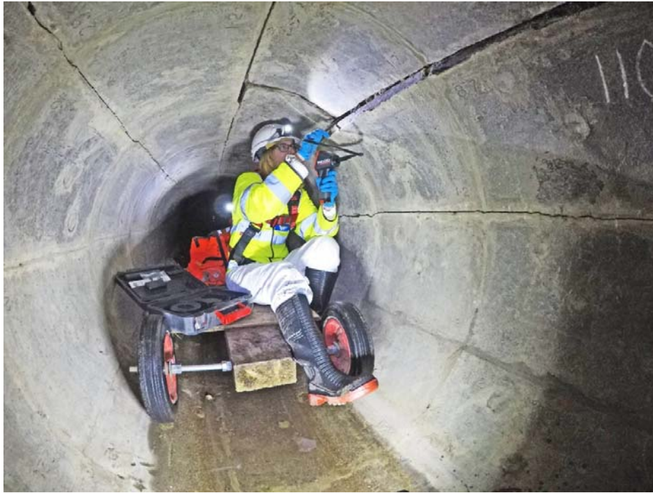
Figure 3. Inspection of open joints by endoscope, confirmed poor original back grouting.
