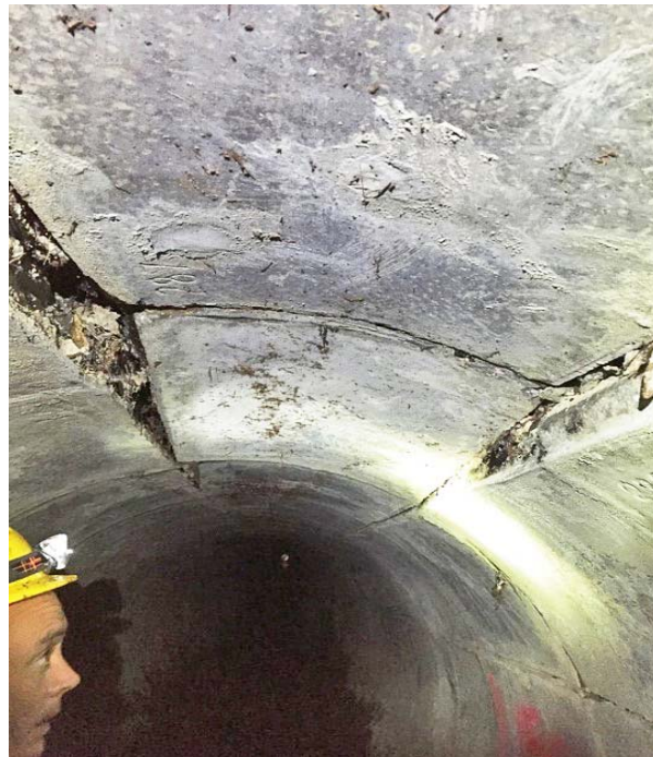
Figure 2. Defects found along the tunnel during person-entry survey.
