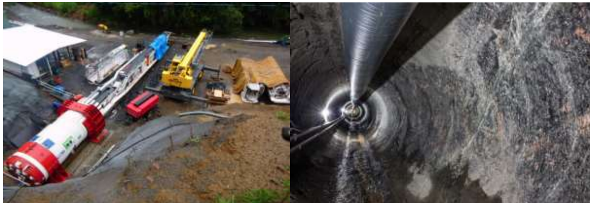
Figure 12 Assembly of the Gripper-TBM ( \varnothing 2850mm) at the starting point of the first tunnel and view in tunnel
