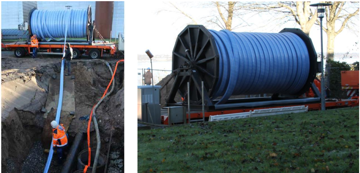
Figure 7: Delivery of the DN 250 PN 15 pre-folded Primus Liner to a construction site
