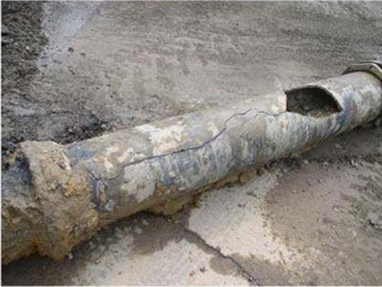
Cast Iron Pipe Broken from Water Hammer
