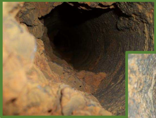
Partial tuberculation removal
