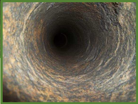
Full tuberculation removal, bitumen liner visible
